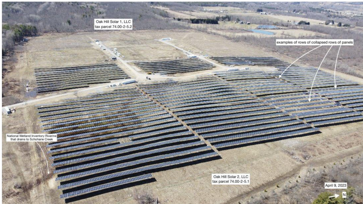
Figure 1. Oak Hill Solar 1, 7.5MW facility in Duanesburg, NY, four months after partial array collapse.
